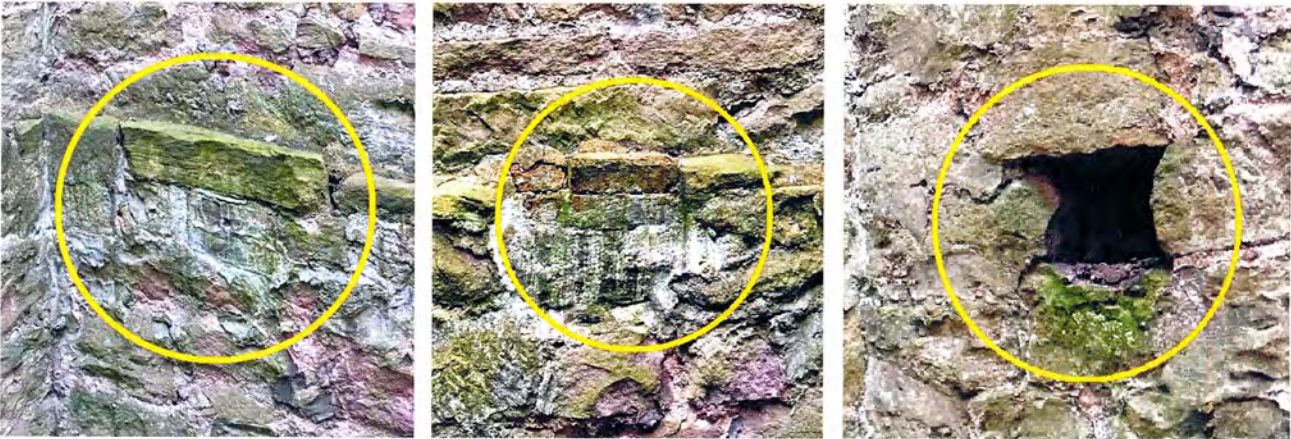
Plate 15 Large c12 inch square beam holes filled, or left open, in the internal north wall.
