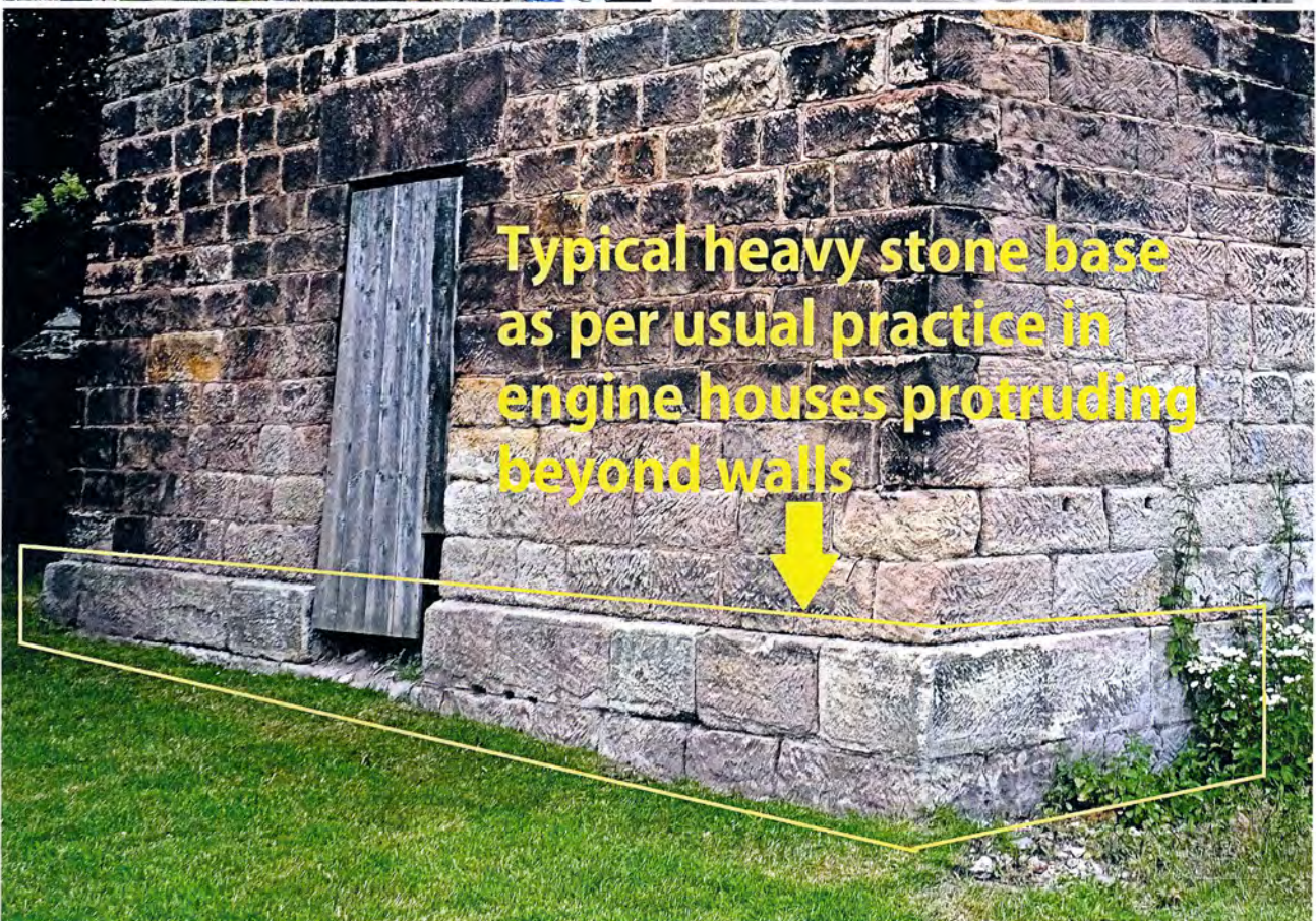
Plate 10 Typical heavy stone base as per usual practice in construction of engine houses protruding beyond walls.
