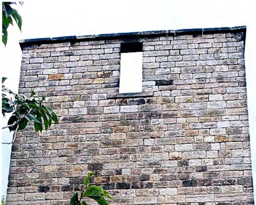
Plate 12 The slotted windows in the north and south walls are suggestive of rope slots rather than for admission of light.
