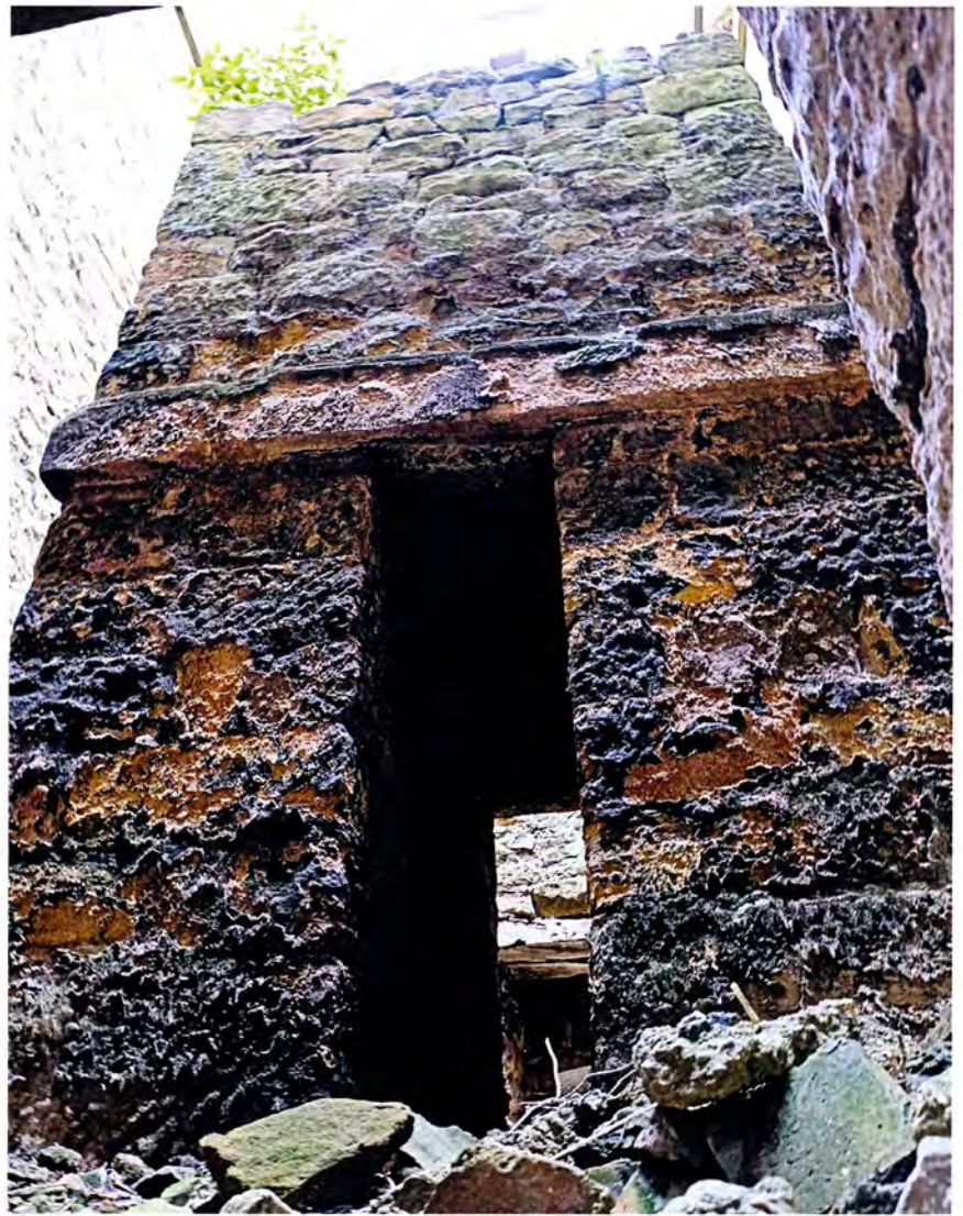
Plate 11 Low angle view from the South doorway of the internal tapered centre column.
